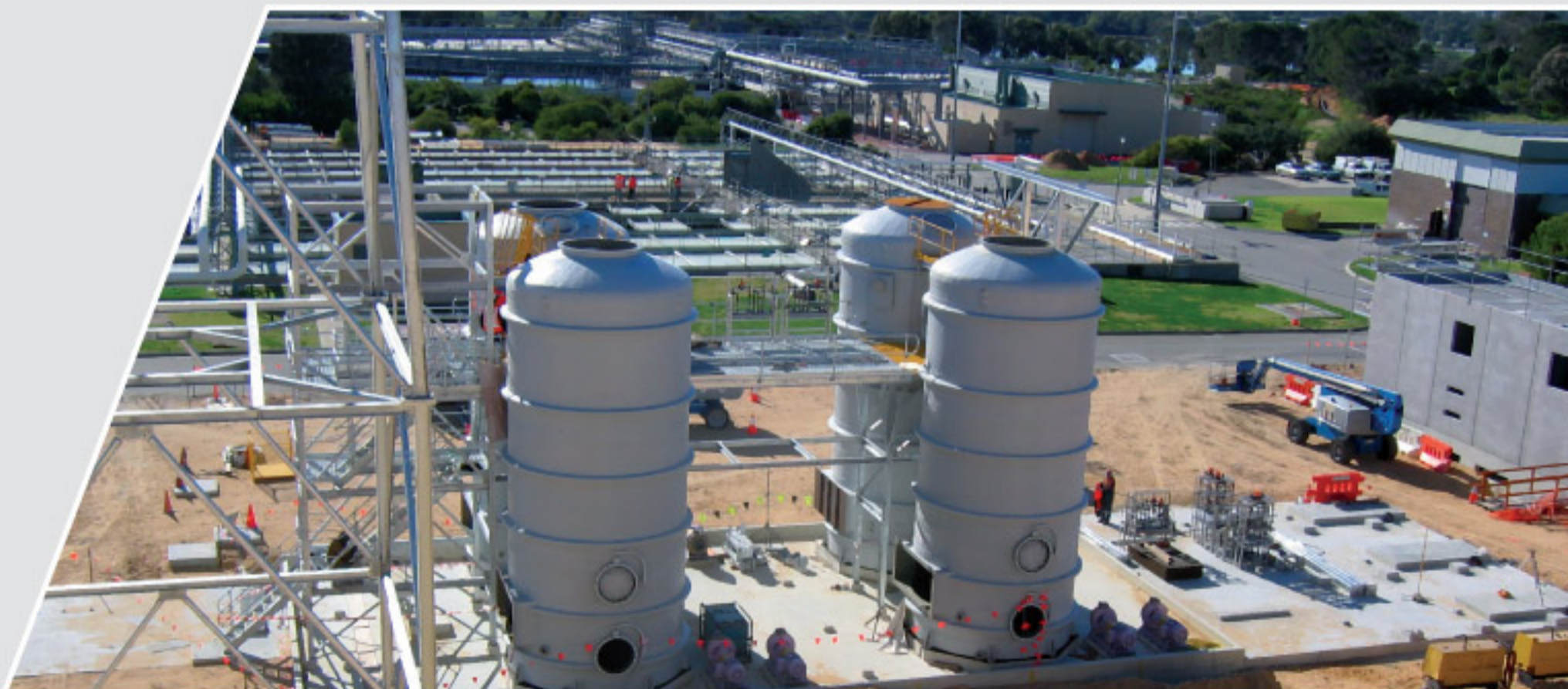
Opposite: Alcoa Pinjarra blow off tank Above: STP Odour Control Unit at Woodman Point
